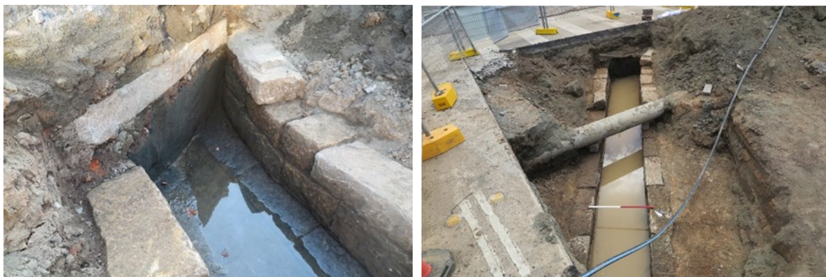
Figure 3.35: Detail of curved eastern wall of Town Drain heading under the pavement of Macquarie Street. View to the north east. IMG_5545 (left). The drain as an effective water receptacle after heavy rain. View to the north east, 1m scale. IMG_5443 (right).
