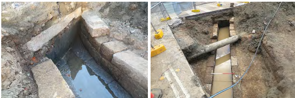
Figure 3.80: Left: Detail of curved eastern wall of Town Drain heading under the pavement of Macquarie Street. View to northeast. IMG_5545. Right: The drain as an effective water receptacle after heavy rain. View to northeast, 1m scale. IMG_5443.
