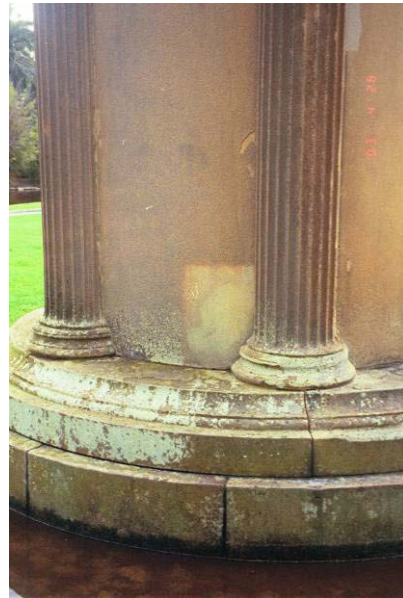
showing rubbed stone at centre, epoxy patch at top right and minimal treatment of base stones, April 2003.
