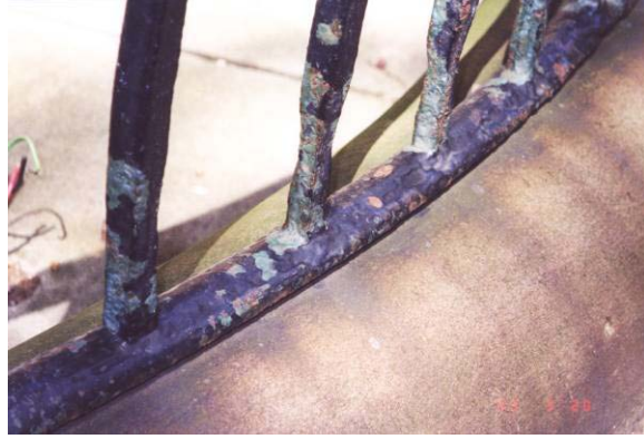
Figure 6.13: Detail of wrought iron balustrade showing loss of paintwork and corrosion, April 2003.
