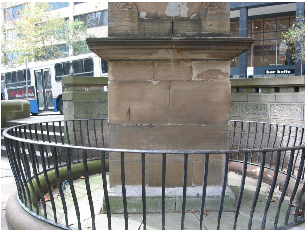
Figure 2.7: Western side of Dado with some damage to the cornice and exfoliation on the base.
