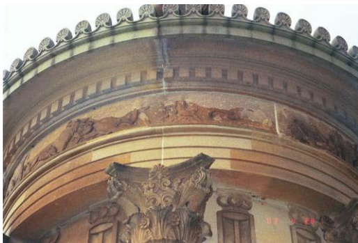
Figure 6.15: Choragic Monument in Royal Botanic Gardens showing sandstone repairs five years after conservation treatment. Stone was replaced in the cornice, while light coloured epoxy patching is evident at the centre of the architrave, April 2003.
