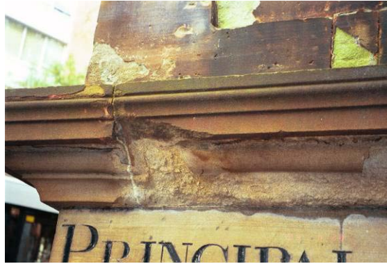
Figure 6.8: Northern cornice showing salt damage, April 2003.
