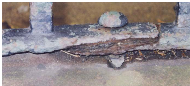
Figure 6.14: Detail of lap join in balustrade showing lead packing at base of bolt and delamination corrosion, April 2003.
